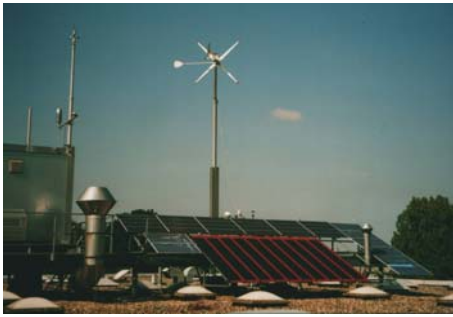
Figure 5: PV installation at the University of Applied Sciences Offenburg.
