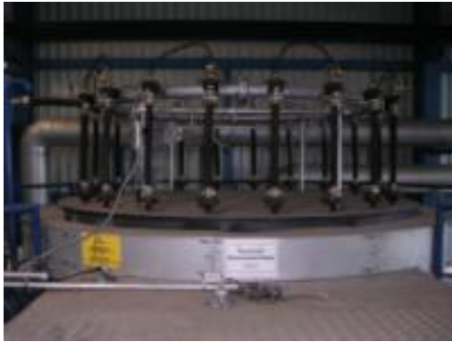
Figure 5: Additional boiler cleaning based on pressurised air.
