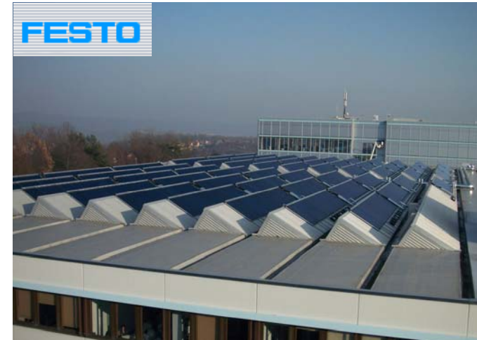
Solar collector field
