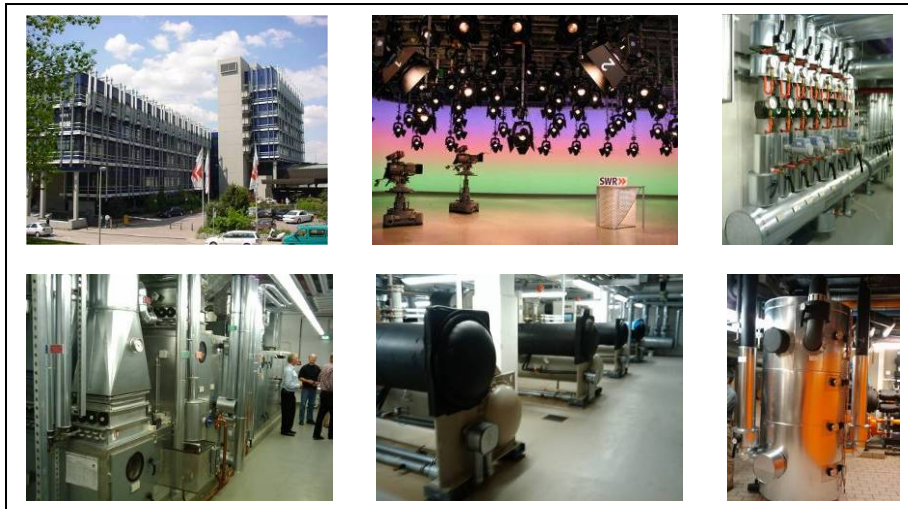
Figure 2: Building view, TV studio and HVAC systems of the SWR buildings in Stuttgart
